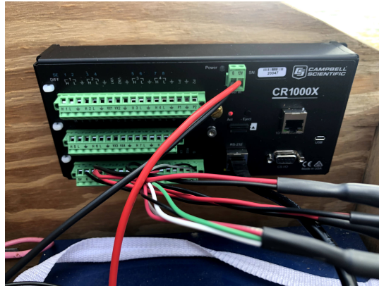
Figure 4: The field setup of the CR1000X data logger used to program and store sensor data.
